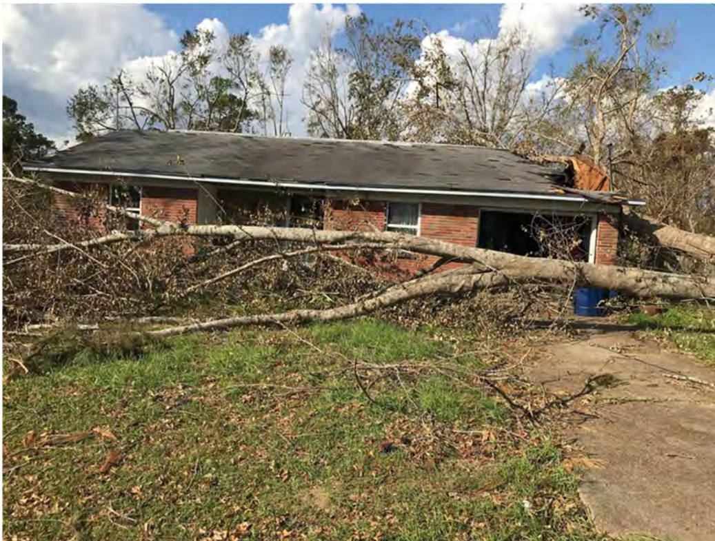
Figure 40: Residential building sustaining severe damage due to tree fall at NE Lambert St. in Blountstown.
