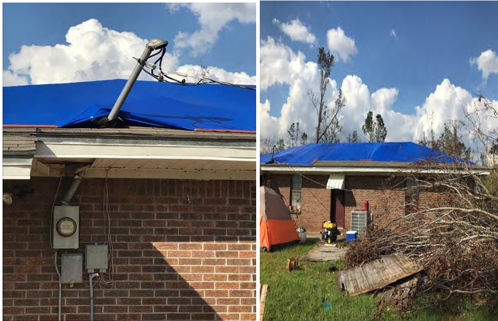
Figure 39: Damaged electricity conductor present in a building near Lambert Ave. in Blountstown.
