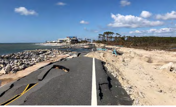
Figure 45: Road washout on Highway 30E (Cape San Blas Rd) on Saint Joseph Barrier Island (Latitude: 29.680619, Longitude: -85.366115).
