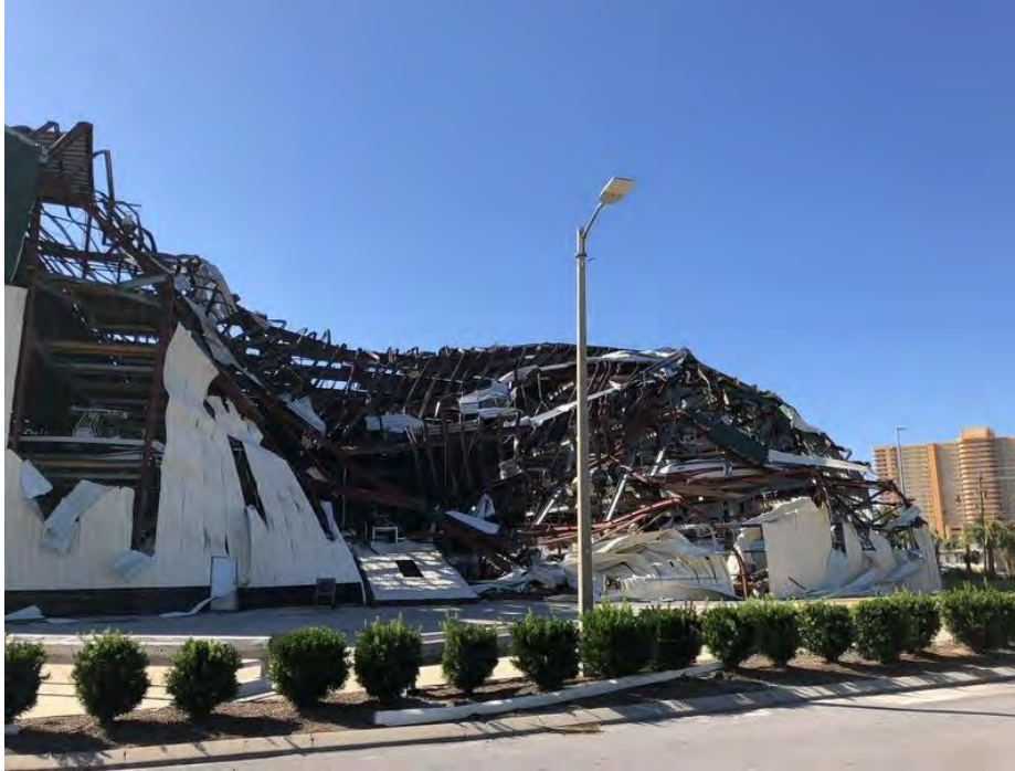
Figure 15: Partial collapse of a metal building marina in Panama City Beach.
