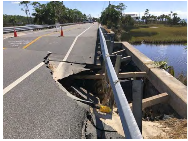
Figure 48: Bridge approach washout on Highway 30A Bridge near Saint Joseph Bay (Latitude: 29.754006, Longitude: -85.303750).
