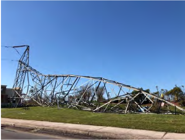
Figure 49: Destroyed transmission tower near North Tyndall Parkway, Springfield (Latitude: 30.160519, Longitude: -85.591164).
