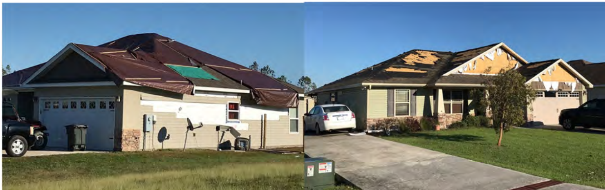
Figure 10: Damage to roof cover and building wall envelope observed in Southport
