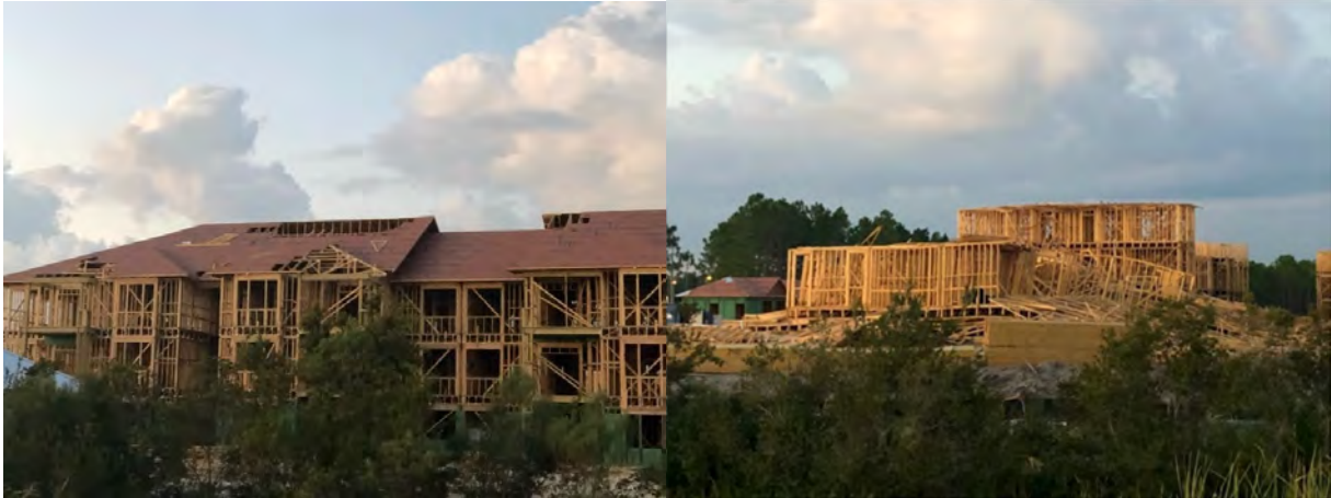
Figure 13: Construction sites in Panama City Beach sustaining moderate wind damage.
