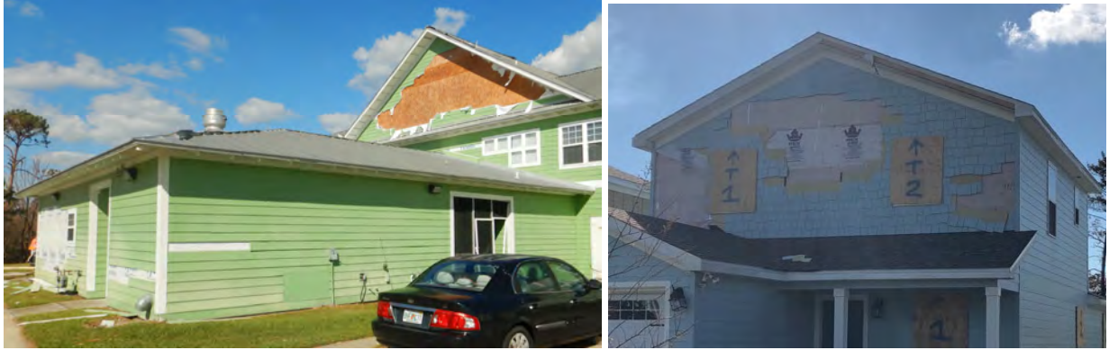
Figure 35: Examples of siding loss in an assisted living facility (left) and single family residence (right) in the Beacon by the Sea community.
