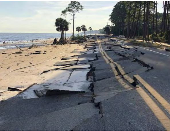
Figure 47: Road washout US Hwy 98 near Carrabelle (Latitude: 29.827057, Longitude: -84.696981) (Source: ESRI StoryMap ).
