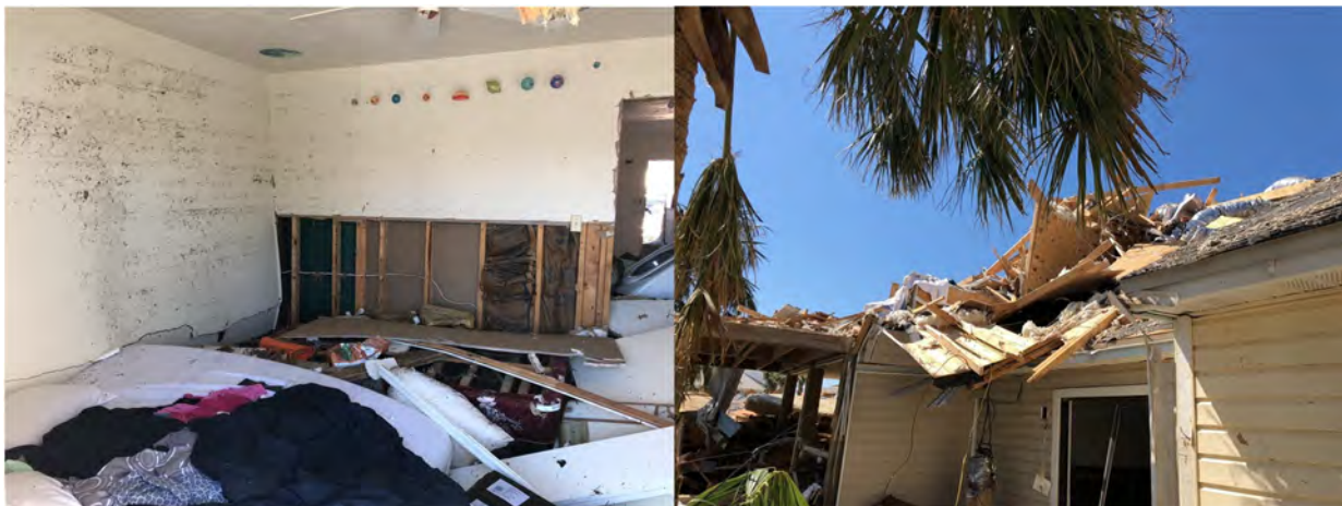
Figure 25: Example of storm surge damage in Mexico Beach. High water mark, 8" short of the 8 ft ceiling, slab is elevated 5" above ground level so surge height estimated 93" AGL.
