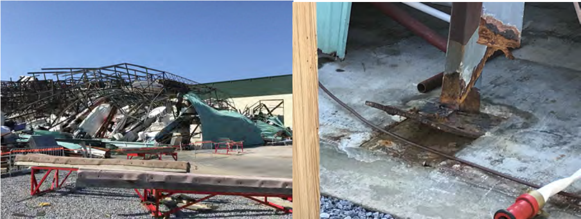
Figure 14: Collapse of a storage building (left) with corrosion and material loss in columns and baseplates (right).
