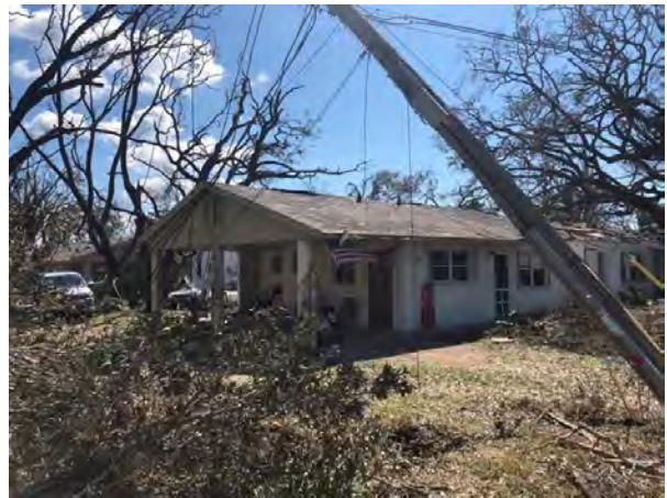
Figure 52: Damaged electric pole near Oakshore Dr., Parker (Latitude: 30.110311, Longitude: -85.60216) (Credit: Dean Ruark)
