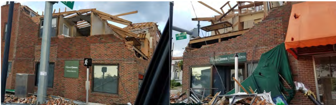
Figure 41: Commercial building (Edward Jones investments) with wall collapsed and roof structure damaged on Lafayette St. in Marianna.
