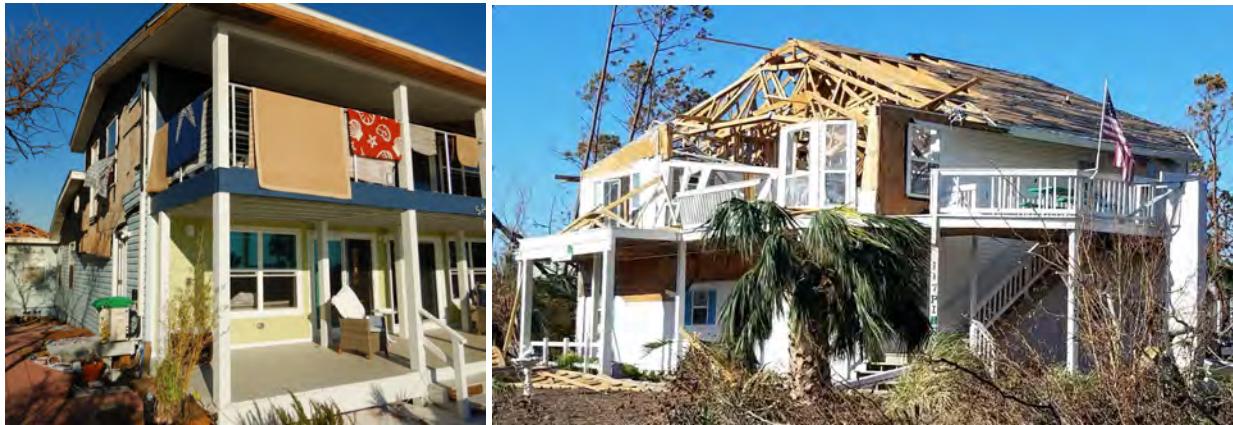
Figure 32: Examples of moderate (left) and severe (right) damage to homes assessed near the intersection of Highways 98 and 386 in Mexico Beach.
