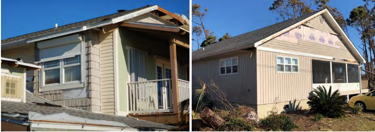
Figure 31: Examples of minor damage to homes assessed near the intersection of Highways 98 and 386 in Mexico Beach.
