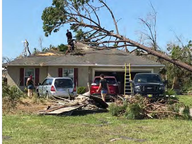
Figure 23: Example of tree damage in Cedar's Crossing.
