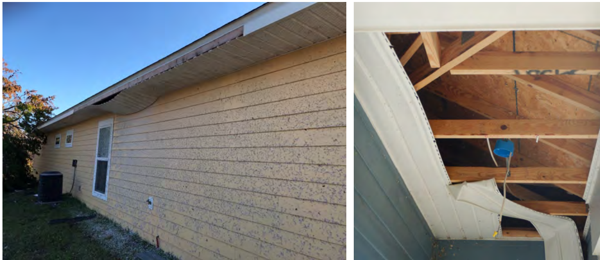
Figure 34: Typical soffit damage to homes in the Beacon by the Sea community.
