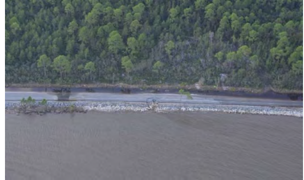
Figure 46: Road wash out US Hwy 98 (Big Bend Scenic Byway Coastal Trail) (Latitude: 29.772736, Longitude: -84.793465) (Source: ESRI StoryMap ).
