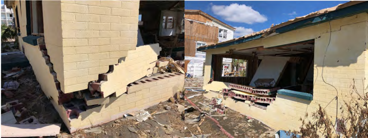
Figure 26: Severe damage to a masonry building observed in Mexico Beach (likely due to storm surge).
