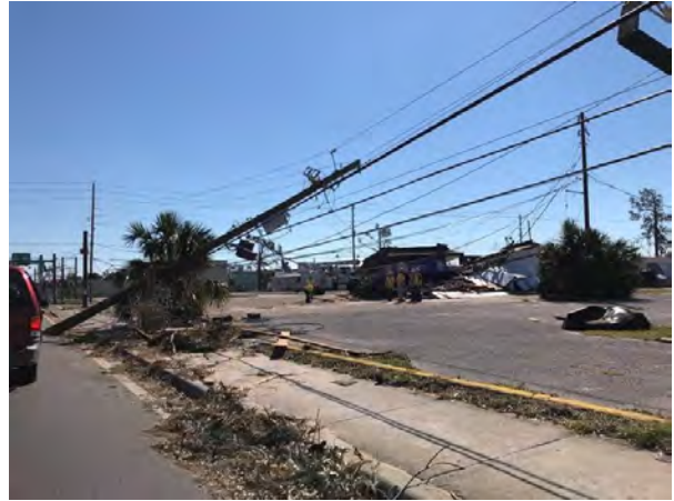
Figure 50: Damaged electric pole near West 15 th St., Panama City (Latitude: 30.175136, Longitude: -85.663061).
