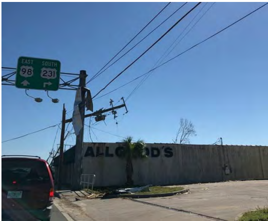
Figure 51: Damaged electric pole near West 15 th St., Panama City (Latitude: 30.175136, Longitude: -85.663061).
