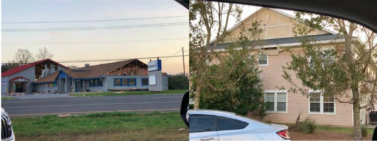
Figure 12: (left) Commercial building in Panama City Beach sustaining severe wind damage. (Right) Multifamily building under construction sustaining minor wind damage in Panama City Beach.
