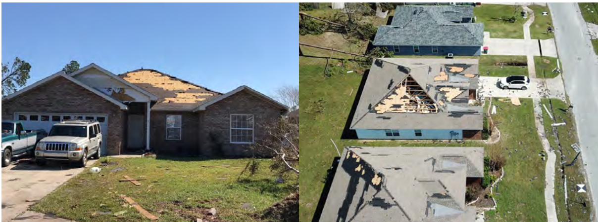
Figure 22: Damage to roof cover and roof sheathing in residential homes in Cedar's Crossing.
