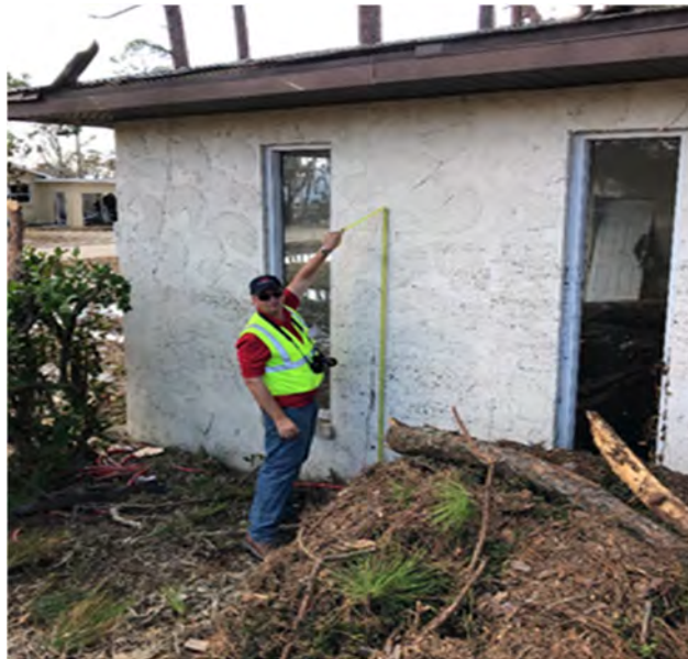
Figure 36: Surge high water mark (72") in Port St. Joe.
