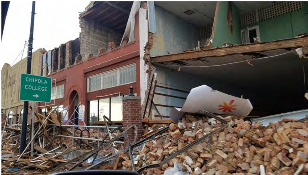
Figure 42: Commercial buildings with masonry walls collapsed and roof structure damage on Lafayette St. in Marianna.
