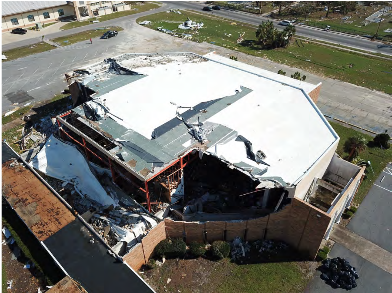
Figure 20: Failure of roof cover and exterior wall of a gymnasium at the Bay County Prep Academy (Lat: 30.16902, Long: -85.67445).
