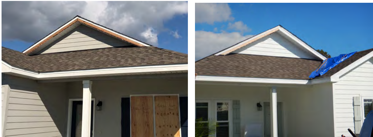
Figure 33: Typical fascia damage of homes in the Beacon by the Sea Community.
