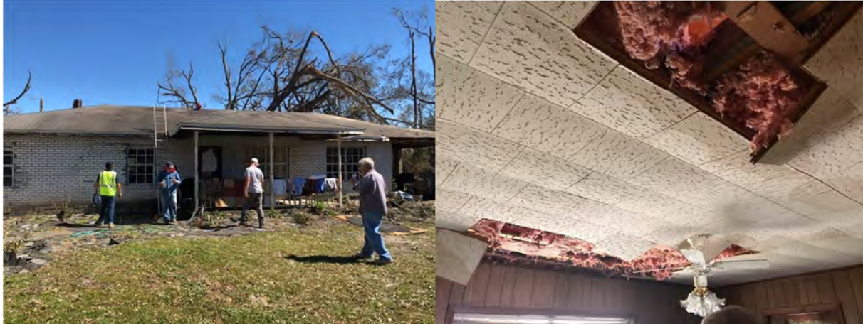
Figure 11: Example of tree damage observed in Southport
