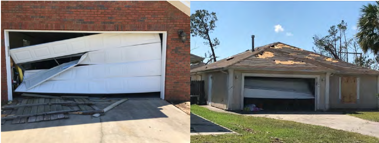
Figure 21: Garage door failures in residential homes in Cedar's Crossing.
