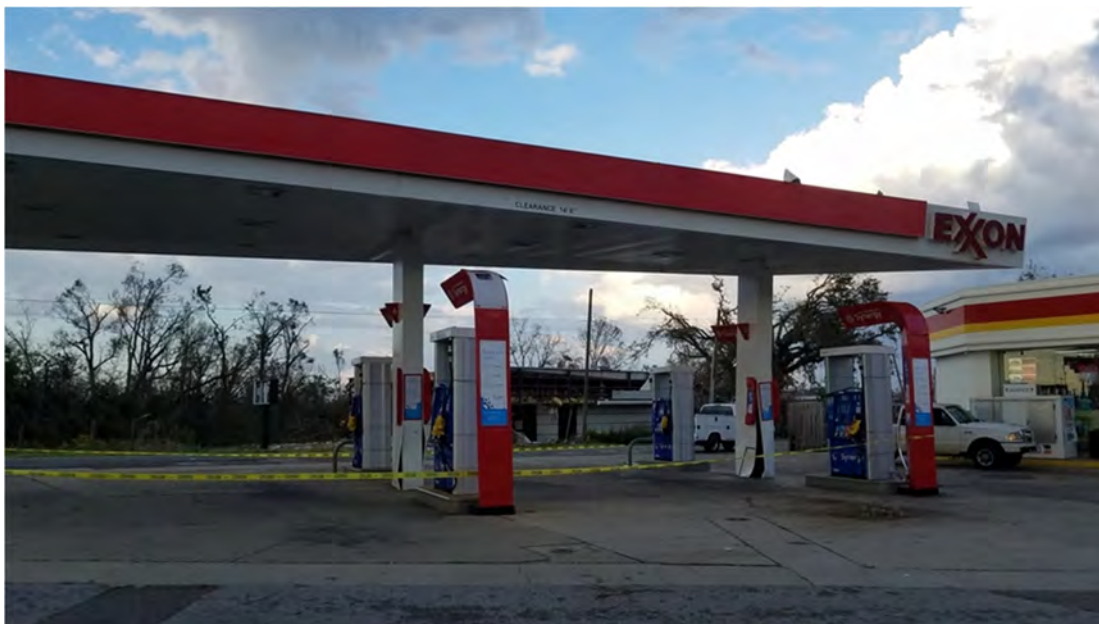
Figure 44: Exxon station sustaining column and roof damage at US 90 in Marianna.
